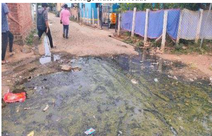
Sewage water on roads
